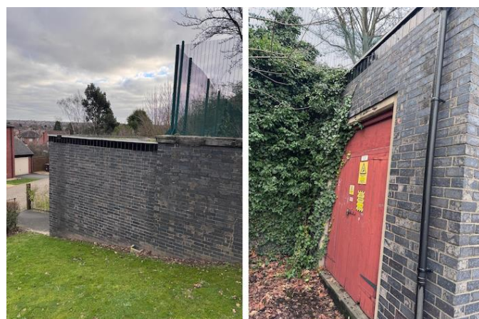
Left: The substation wall that is being used as a climbing frame. Right: The overgrowth after it was cut back.
